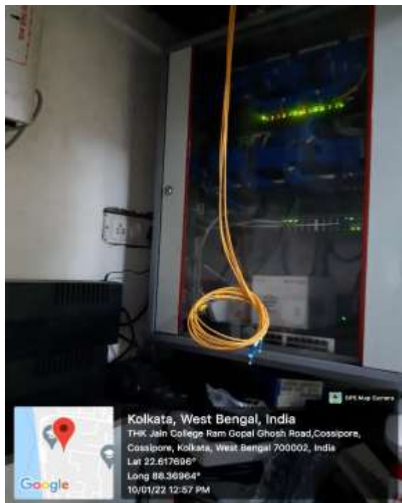
The main server for WiFi connection
