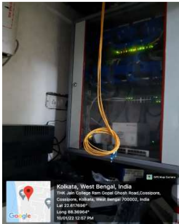
The main server for WiFi connection
